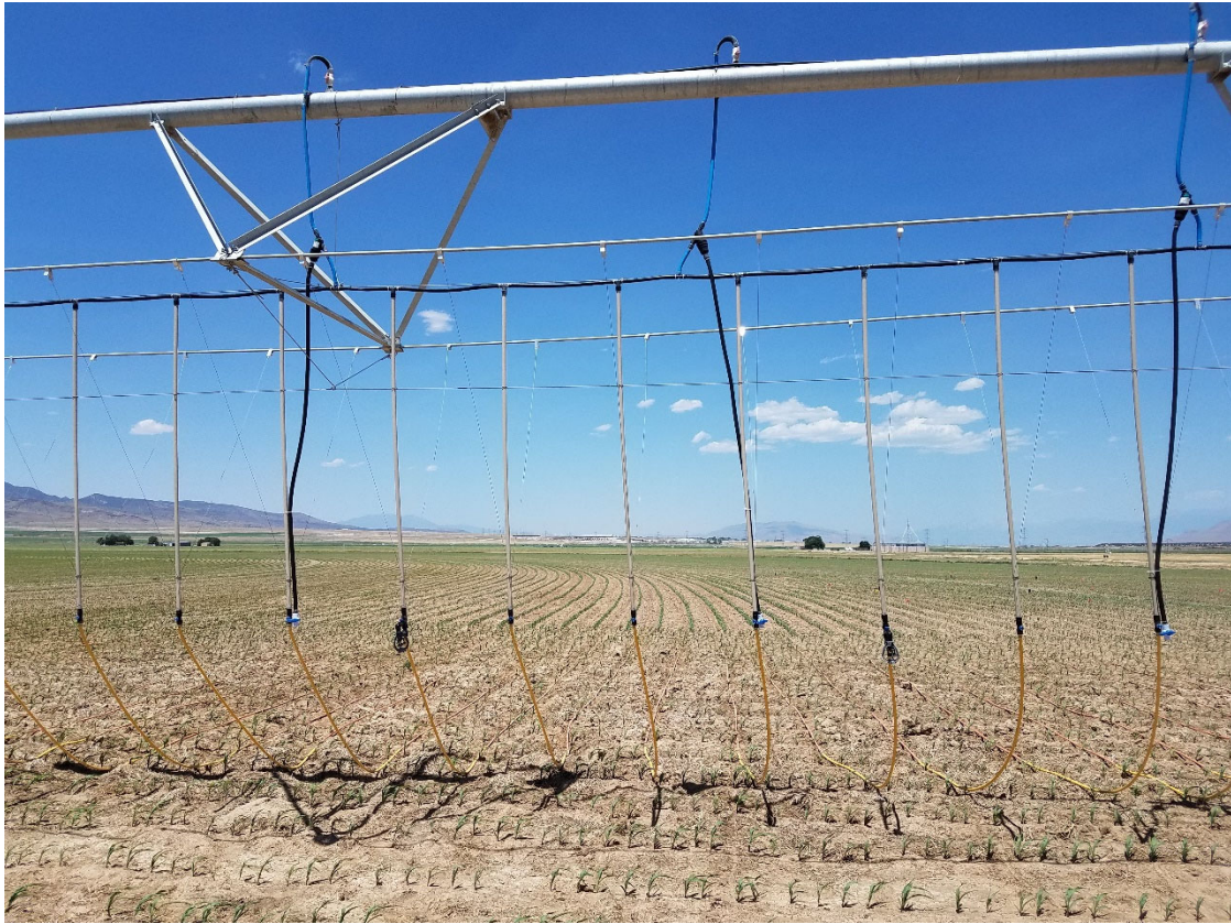
Figure 3. The filters can be seen on the feed lines from the pivot pipe above. Whole system filtration near the pump is recommended if the entire pivot uses MDI. The ties used to keep the rigid drops vertical can also be seen secured to the truss rods.
