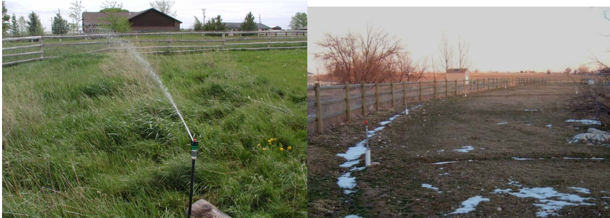
Figure 8. (left) Nelson R2000 “windfighter” nozzle; (right) Nelson R2000 sprinklers in a solid-set arrangement with buried main and submains and risers protected by PVC pipe.
