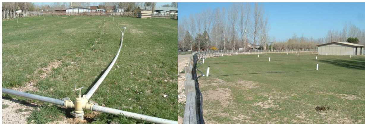
Figure 5. (left) Solid-set sprinkler lines for irrigation of horse pasture; (right) Semi-permanent solid-set sprinkler heads connected by plastic tubing with laterals connected to mainline by quick-couple connectors.
